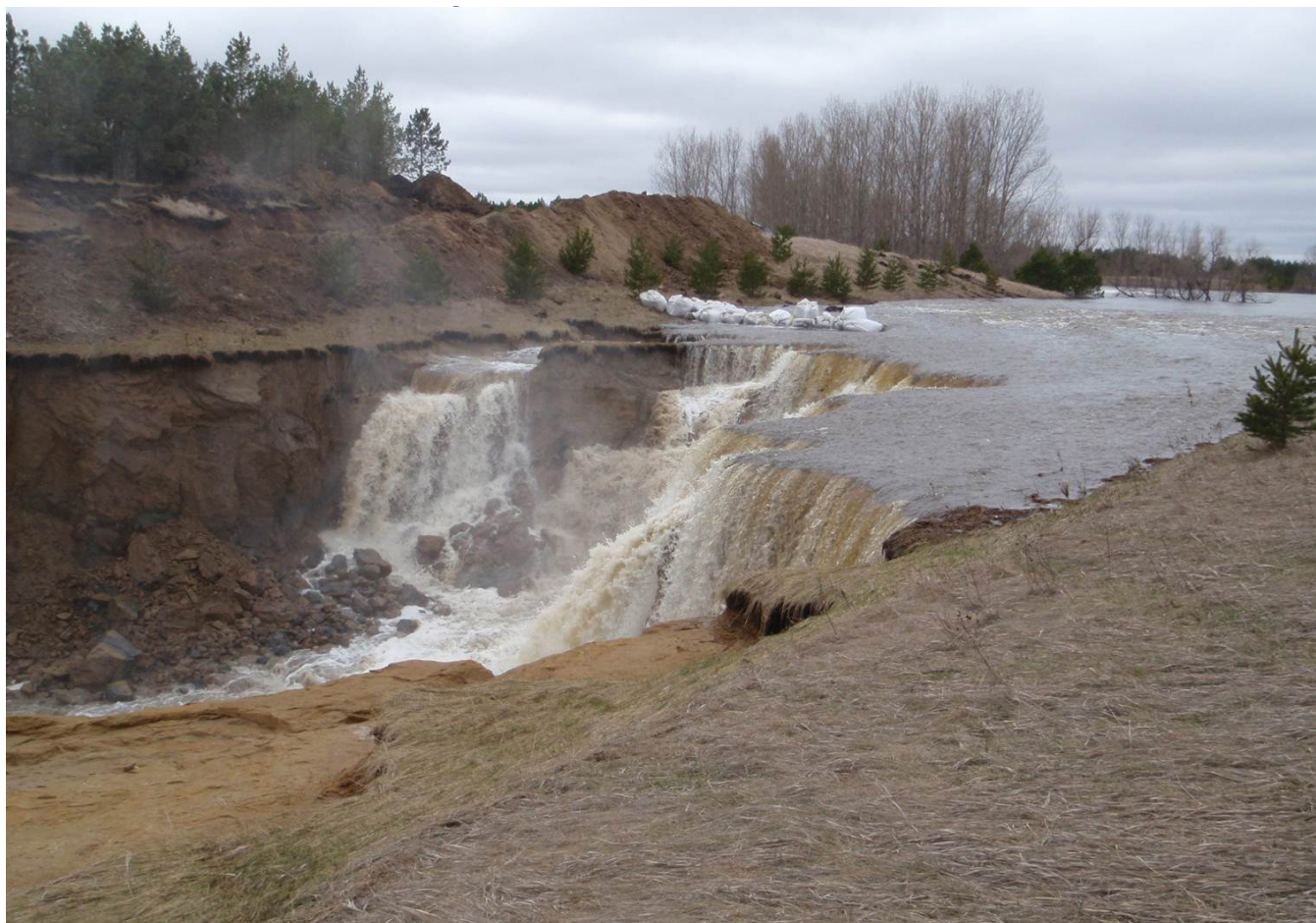
Figure 9: Severe Auxiliary Spillway Erosion
