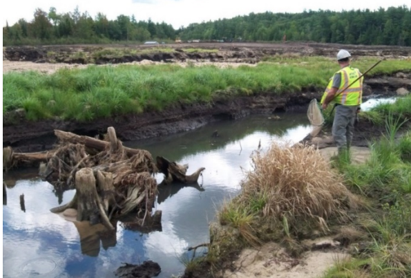
Figure 9: Construction staff rescue stranded fish during dewatering and transport fish back to the main channel.
