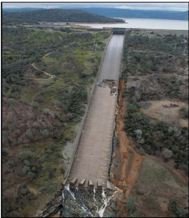
Figure 15. Initial Damage Sustained at Oroville Dam Service Spillway (February 7, 2017) [1].
