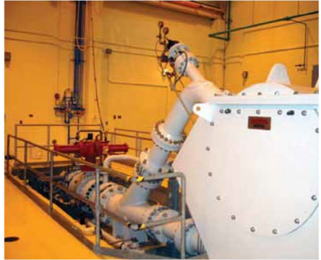
Figure 6. Lakewood Reservoir Dam Pipeline Hydroelectric Powerhouse
