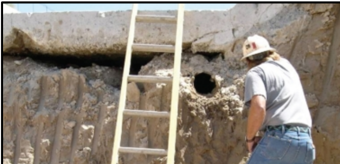
Figure 5. Foundation Erosion under Spillway Chute Slab due to Migration of Material through Unfiltered Drains [9].
