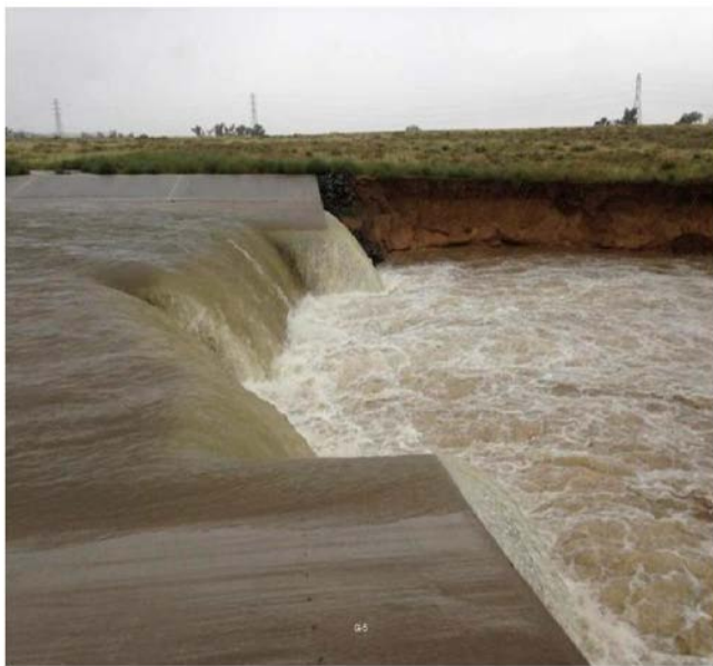
Figure 11. Headcut Eroding Spillway at Havana Street Dam.
