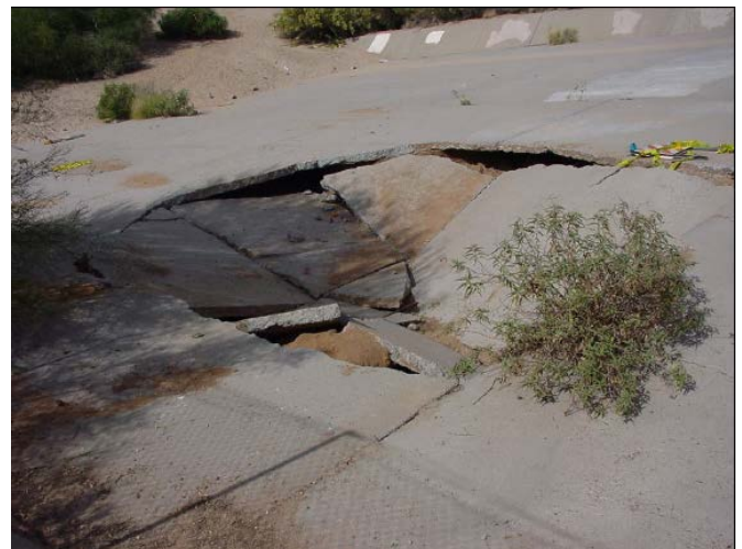
Figure 3. Brittle Collapse of Unreinforced Slab System due to Foundation Erosion [10].
