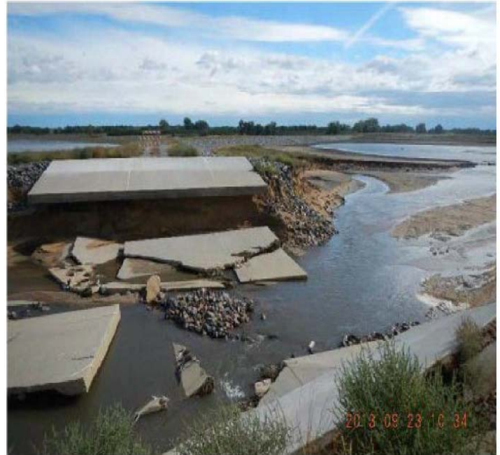
Figure 12. Breached Spillway at Havana Street Dam.
