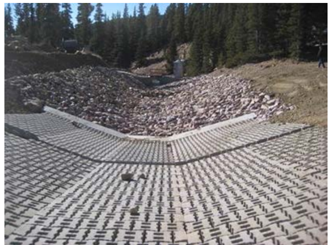
Figure 2. ACBs (foreground) and riprap (background) lining a spillway chute at a dam in Colorado.
