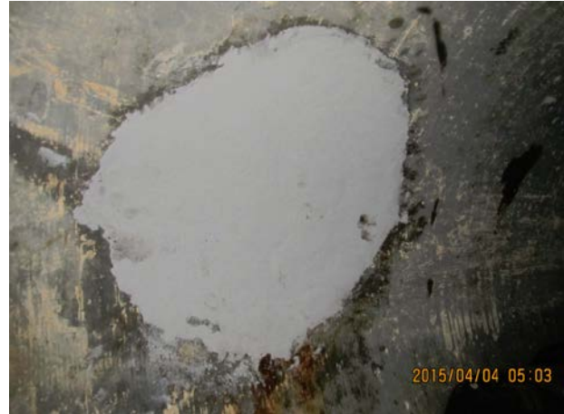
Figure 8. Patch repair of pipe wall damage prior to mechanical seal installation (photo courtesy of NRCS).
