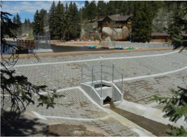
Figure 7. Downstream Face of Grace Lake Dam after Installation of ACB Overtopping Protection.
