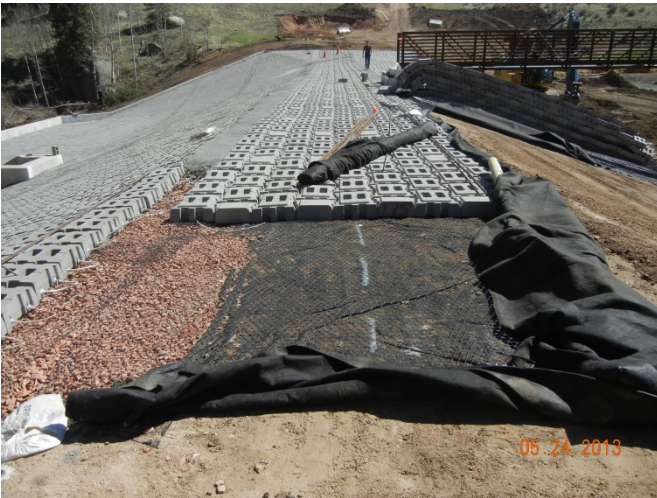
Figure 8. Placement of ACB Mats on the Crest and Downstream Slope of Leo Dam (looking northeast).
