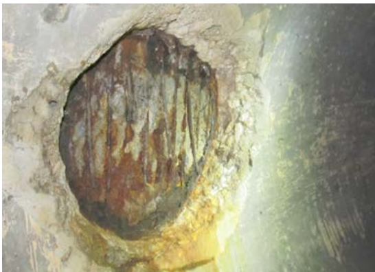
Figure 7. Hole through Pipe Wall (photo courtesy of NRCS).
