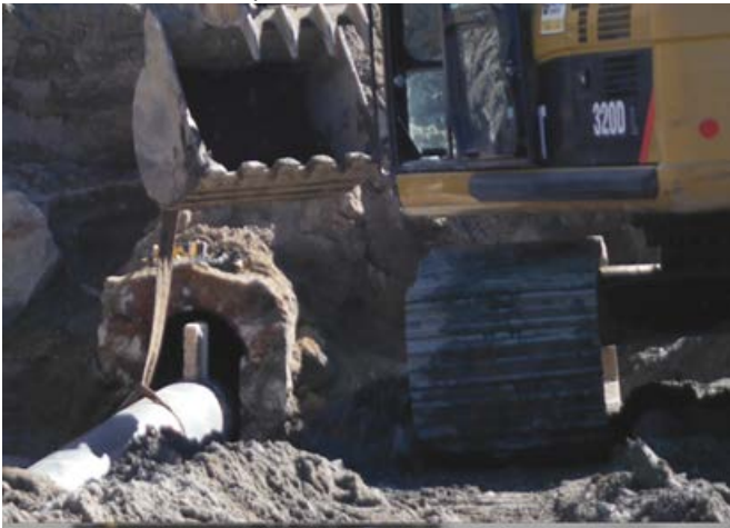
Figure 2. Conduit Sliplining with Relatively Large Annular Space Prior to Cellular Grout Placement at Estler Lake Dam
