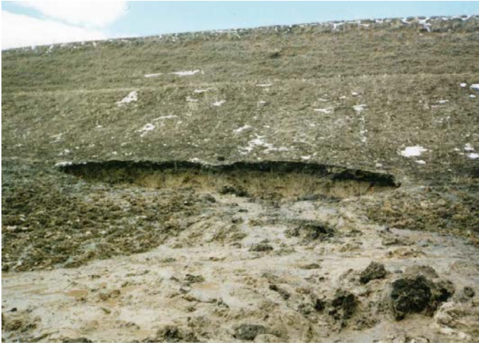
Figure 4. “Blowout” Caused by Underseepage of a Dam in Montana (MT DNRC)
