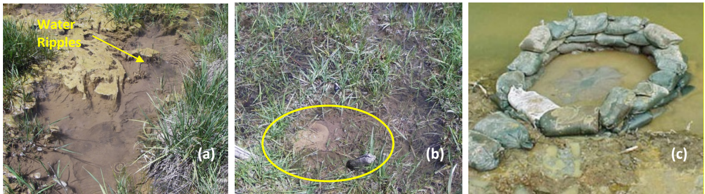
Figure 11. Sand boils on downstream toes are often slightly submerged, and sometimes detectable by water ripples (a). They may start as very small deposits (b). Once observed they are often sandbagged to help limit progression (c).
