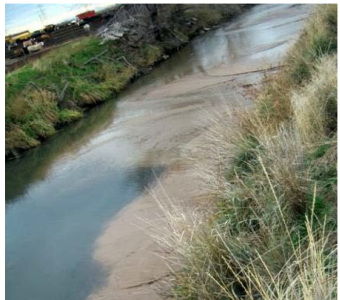
Figure 10. Sediment Plume within a Drainage Ditch along the Downstream of a Dam Toe [2]
