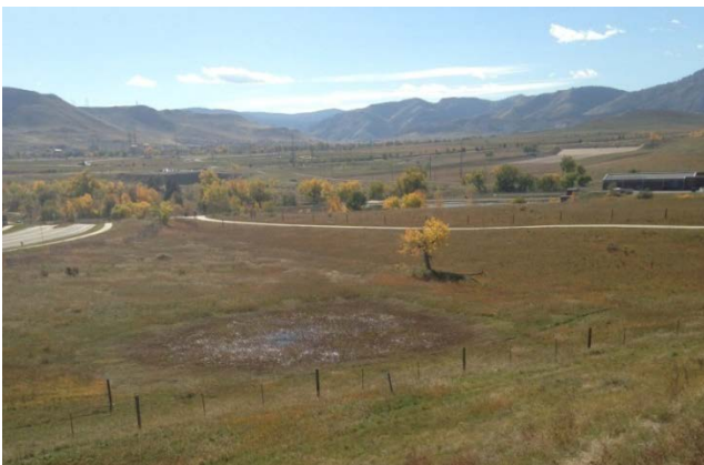
Figure 7. Underseepage at Dam Toe at a Colorado Dam
