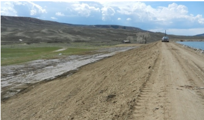
Figure 6. Underseepage at Dam Toe Rising to Surface (Wyoming NRCS)
