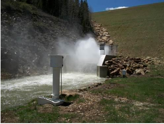
Photo 1: Releasing 300 ft 3 /sec through a Low Level Outlet at Dam in Utah
