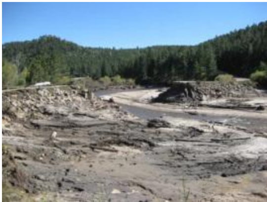
Photo 9: Mirror Lake Dam post-failure looking downstream from left abutment.
