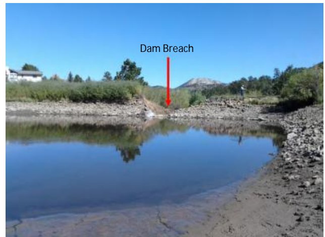
Photo 12: CH2 Dam post-failure looking downstream from reservoir. Note heavy vegetation on dam crest.
