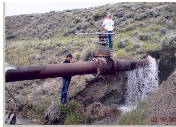
Photo 6. Damage Incurred to Outlet Conduit during Operation
