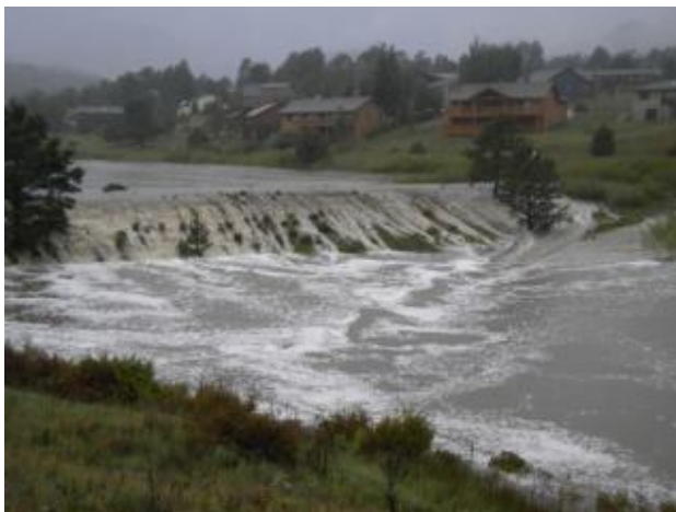
Photo 14: CH1 Dam overtopping.
