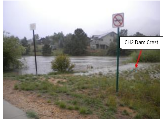
Photo 15: CH2 Dam overtopping.
