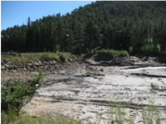
Photo 8: Willow Lake Dam post-failure looking downstream near left abutment.
