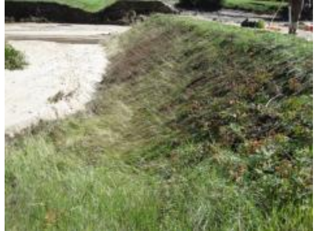
Photo 6: Downstream slope of Sunset Lake Dam after overtopping looking from left abutment.
