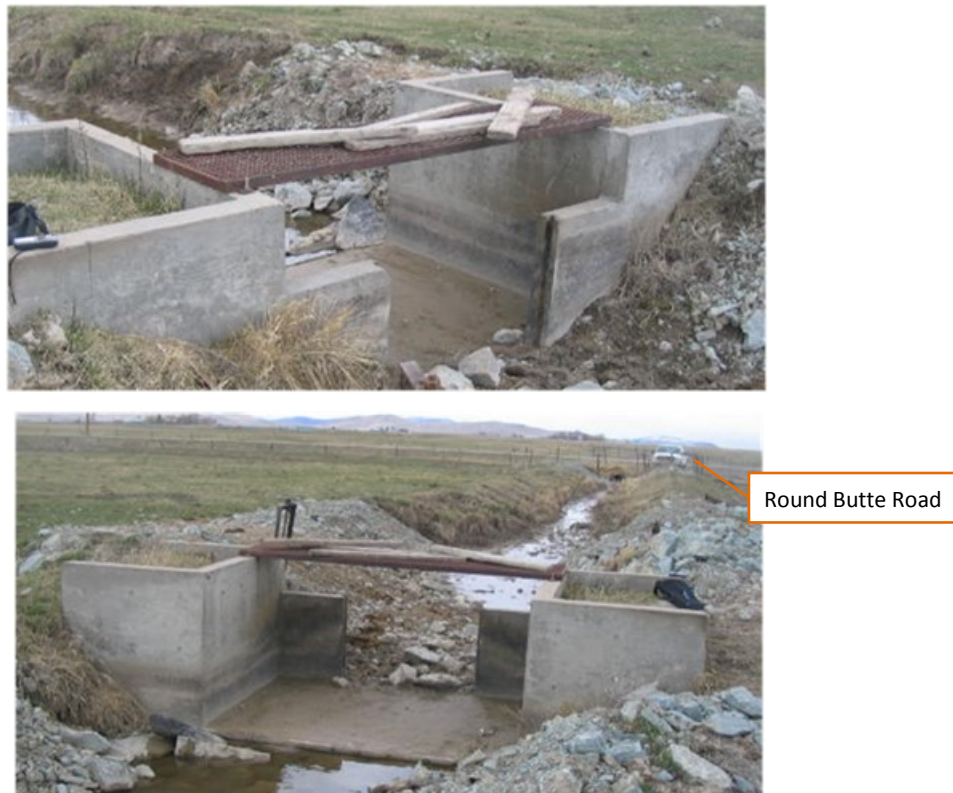
Figure 28. Upstream view (top) and downstream view (bottom) of the existing check structure in Sub-Lateral 50A-19-1 at Round Butte Road. Photos from HKM 2008 report.
