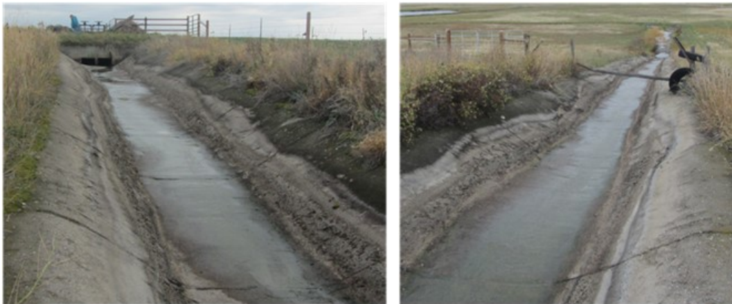
Figure 10. Upstream view (left) and downstream view (right) of chute drop immediately downstream of the Lateral 73A headgates
