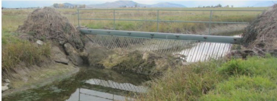
Figure 7. Existing trash rack in the Pablo A Canal just downstream of the inlet to Horte Reservoir. Notice the large piles of aquatic debris on the canal banks and on the screen itself.
