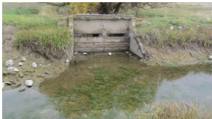
Figure 6. Existing spill structure to maintain water level in the Pablo A Canal and pass all excess flows to Horte Reservoir
