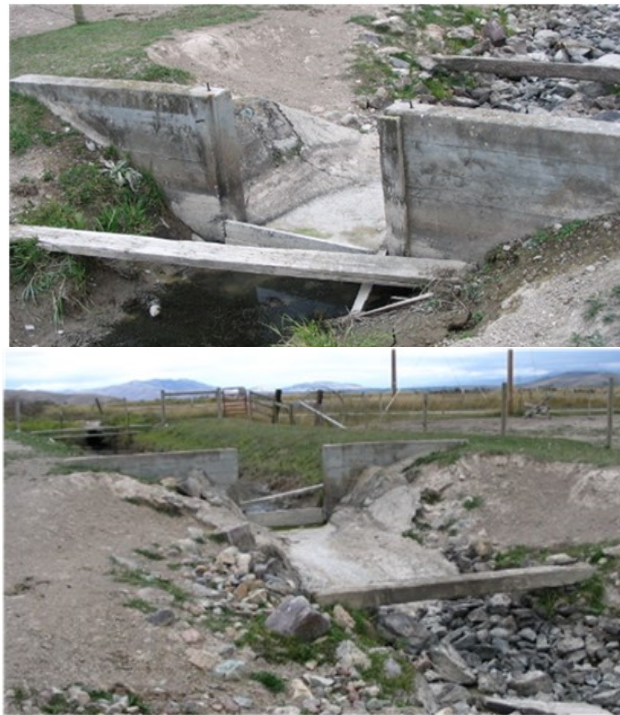
Figure 57. Upstream view (top) and downstream view (bottom) of the existing check structure in Lateral 73A downstream of Beaver Drive. Photos from HKM 2008 report (CD-71).
