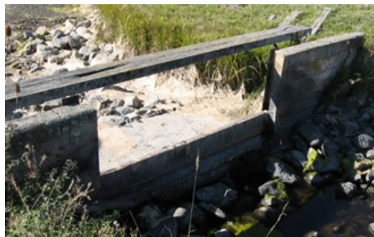
Figure 67. Existing check structure at the head of Sub-Lateral 73A-5. Photo from HKM 2008 report (CH-387).
