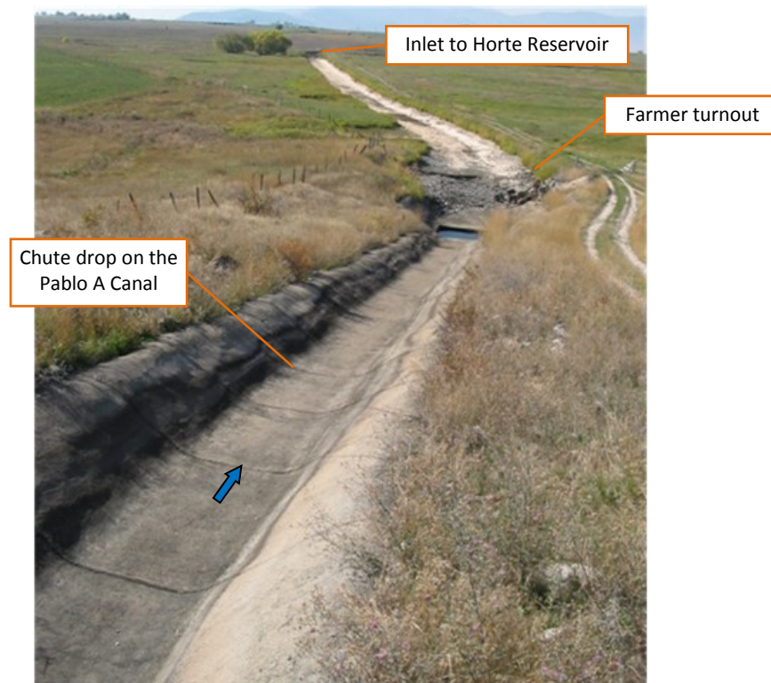
Figure 5. Existing chute drop on the Pablo A Canal several hundred feet upstream of inlet to Horte Reservoir. Photo from HKM 2008 report (CHT-11).
