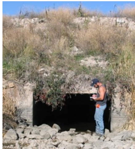
Figure 48. Lateral 70A headgate discharge. There appears to be large elevation drop across the headgate. Photo from HKM 2008 report (CHT-11).
