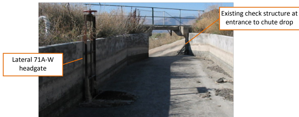
Figure 4. Existing check structure at entrance to chute drop on the Pablo A Canal several hundred feet upstream of inlet to Horte Reservoir. Photo from HKM 2008 report (CHT-11).
