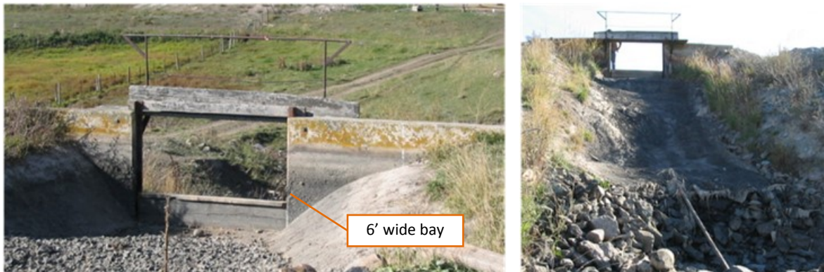
Figure 66. Existing check drop at the head of Sub-Lateral 73A-4. Photo from HKM 2008 report (CD-82).
