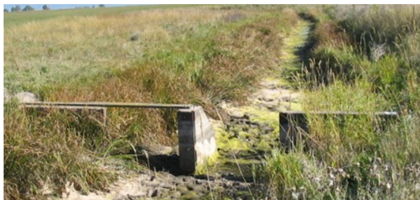
Figure 49. First existing check structure on Lateral 70A. Photo from HKM 2008 report (CH-351)
