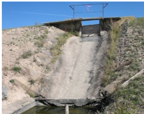
Figure 68. Downstream view of existing check drop at the head of Sub-Lateral 73A-4. Photo from HKM 2008 report (CD-79).
