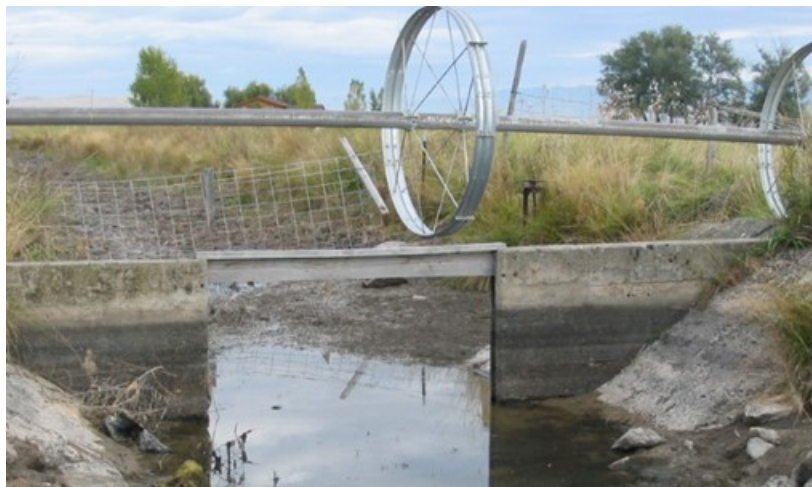
Figure 35. Existing check structure in Lateral 70A immediately downstream of the Sub-Lateral 70A-19 headgate. Photo from HKM 2008 report (CH-368). The side roll sprinkler lateral appears to be lost.
