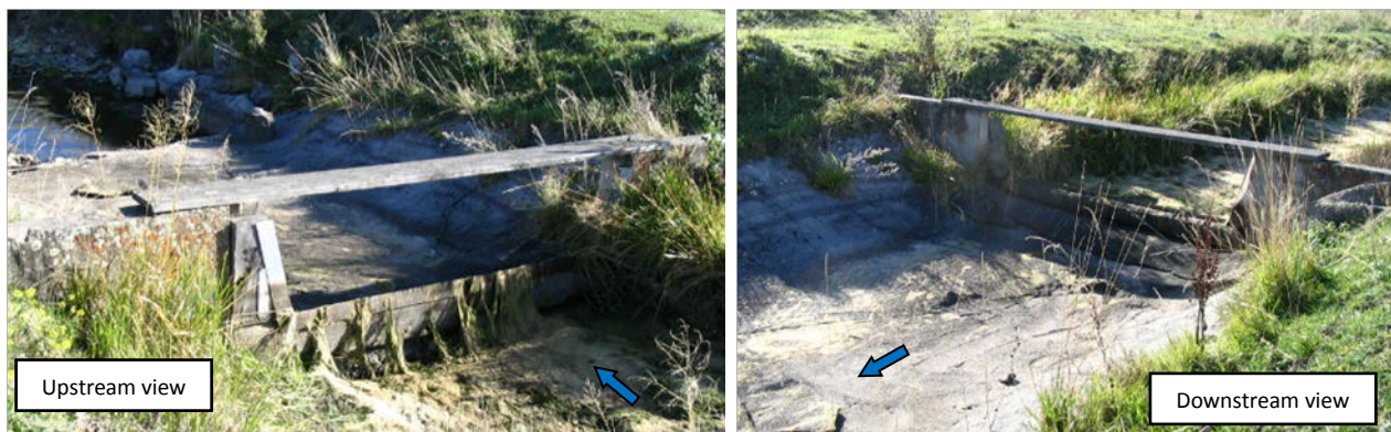
Figure 13. Existing Cipoletti weir in Sub-Lateral 31A-1. Photos from HKM 2008 report.
