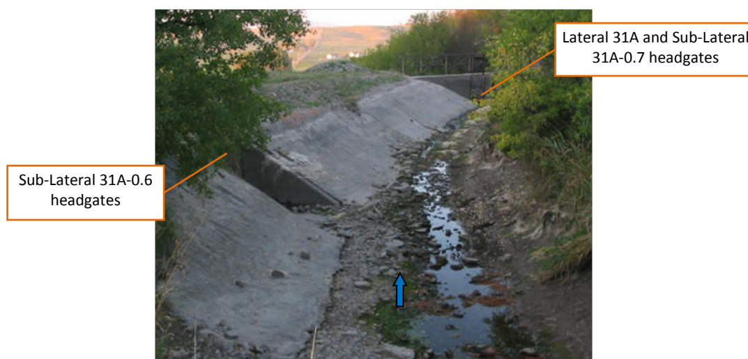
Figure 4. Existing lateral headgates in pool downstream of the Valley View Tunnel discharge. Photo from HKM 2008 report.
