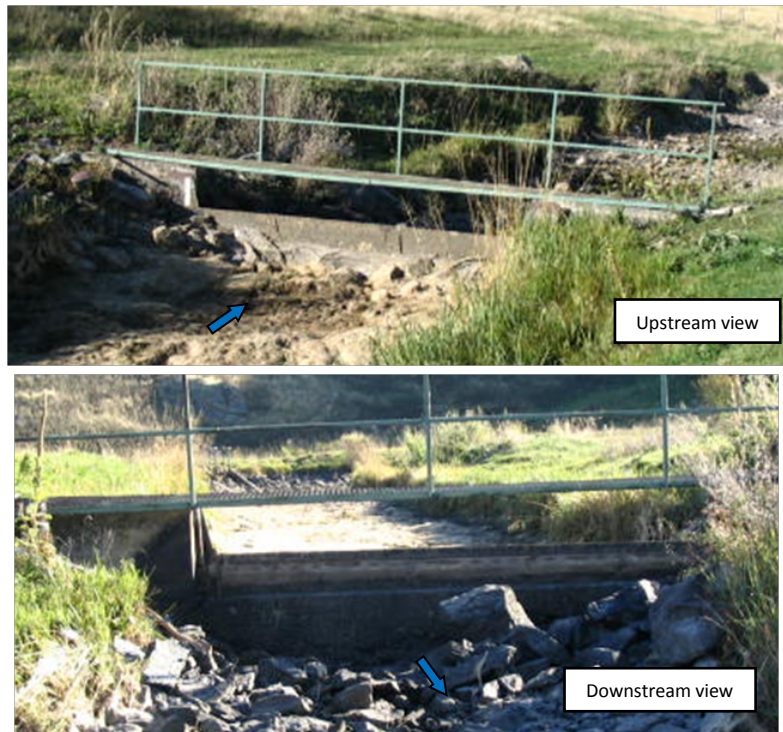
Figure 12. Existing Lateral 31A Cipoletti weir used for flow measurement and water level control for Sub-Lateral 31A-1 headgate located upstream. Photos from HKM 2008 report.
