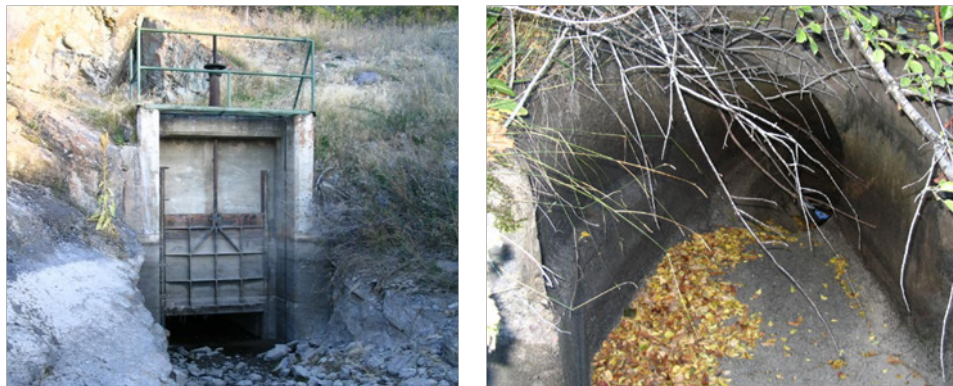
Figure 3. Existing sluice gate at the entrance to the Valley View tunnel (left) and tunnel discharge (right). Photos from HKM 2008 report.
