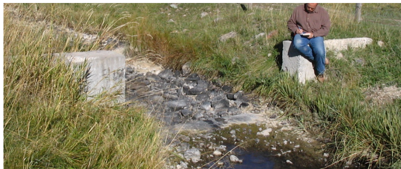
Figure 21. Existing check structure in Lateral 31A downstream of the Sub-Lateral 31A-30 headgate. Photo from HKM 2008 report.
