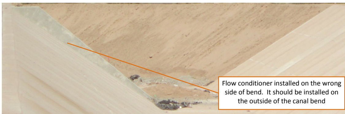
Figure 39. Examples of flow conditioner walls. Note the photo on the bottom has the flow conditioner constructed on the wrong side of the canal. The conditioner must be constructed on the outside of a canal bend.
