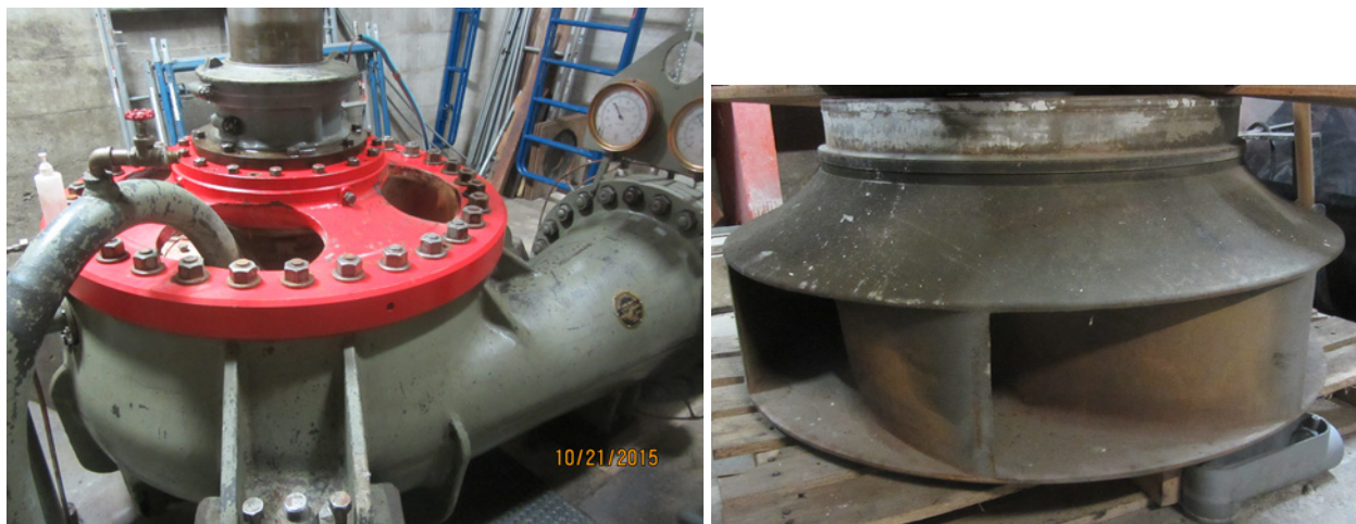
Figure 5. Single stage vertical centrifugal pump (left). Old impeller with pitting that needs to be repaired (right).
