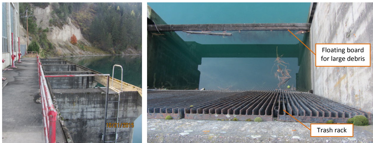
Figure 3. Pump house intakes on the Flathead River
