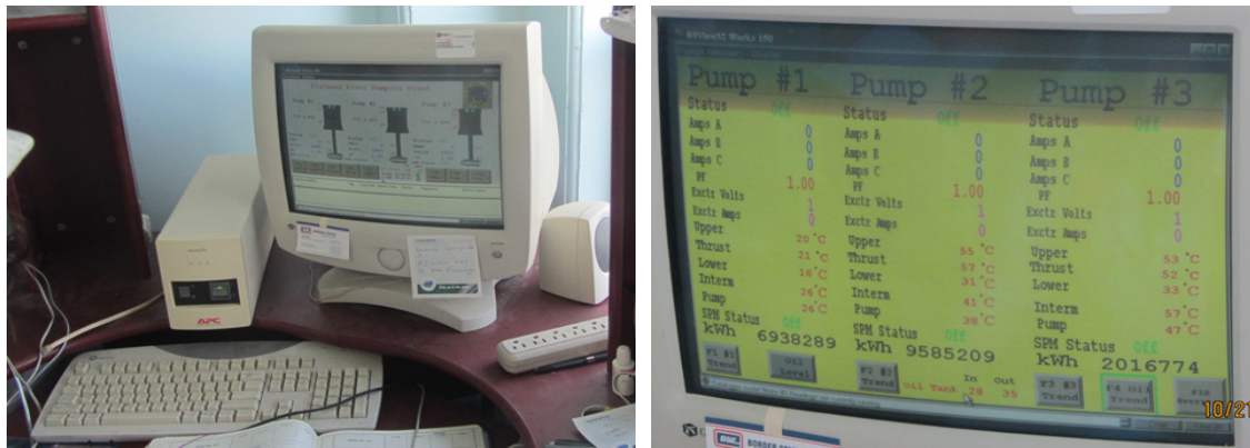
Figure 6. Existing SCADA system for the river pumps
