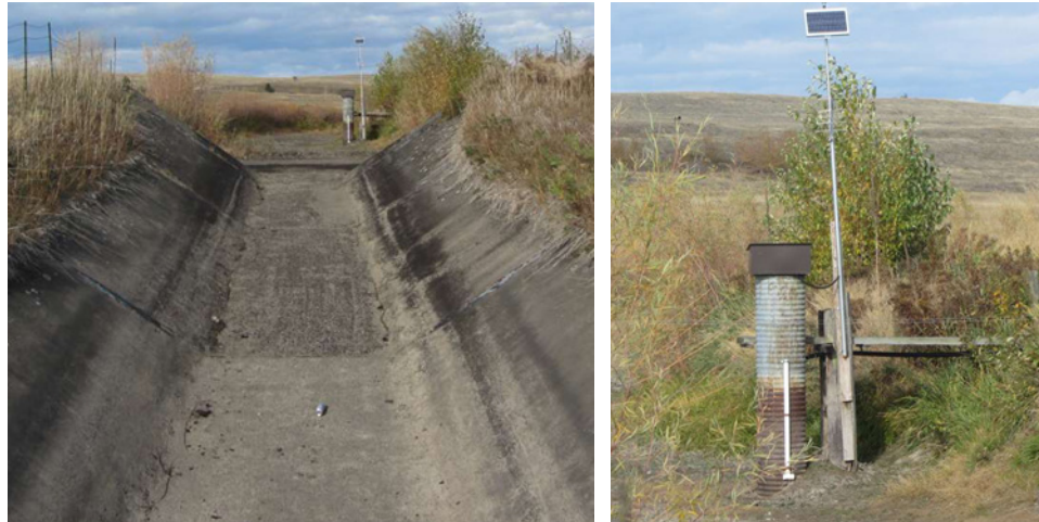
Figure 15. Existing GOES gauging station upstream of the Pablo Drop
