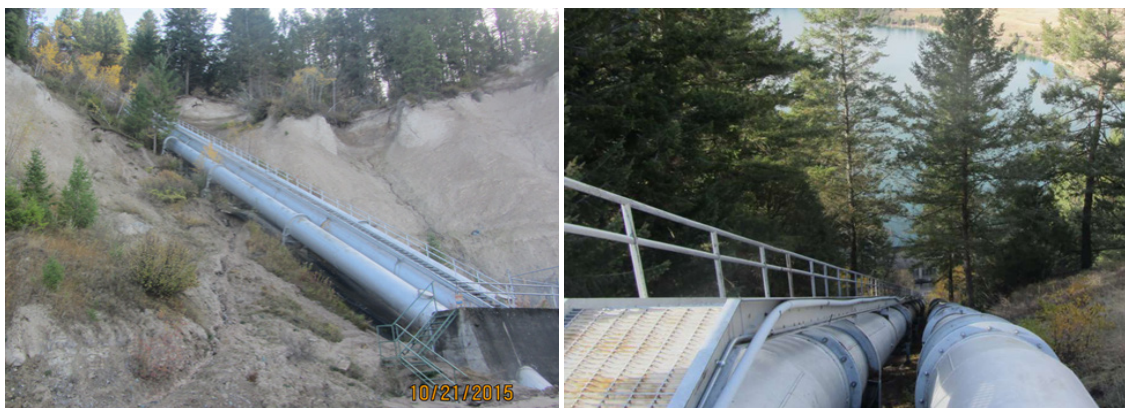
Figure 7. Pump discharge pipelines
