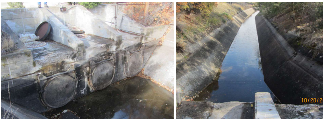
Figure 8. Discharge into the Pump Canal
