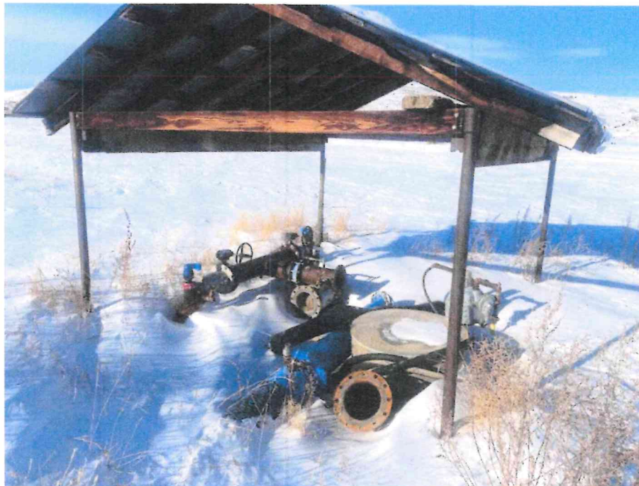
Figure 4: Intakes of buried pipelines at pump site in the SWNWSE of Section 5, T5S R20E, December 16, 2022.
