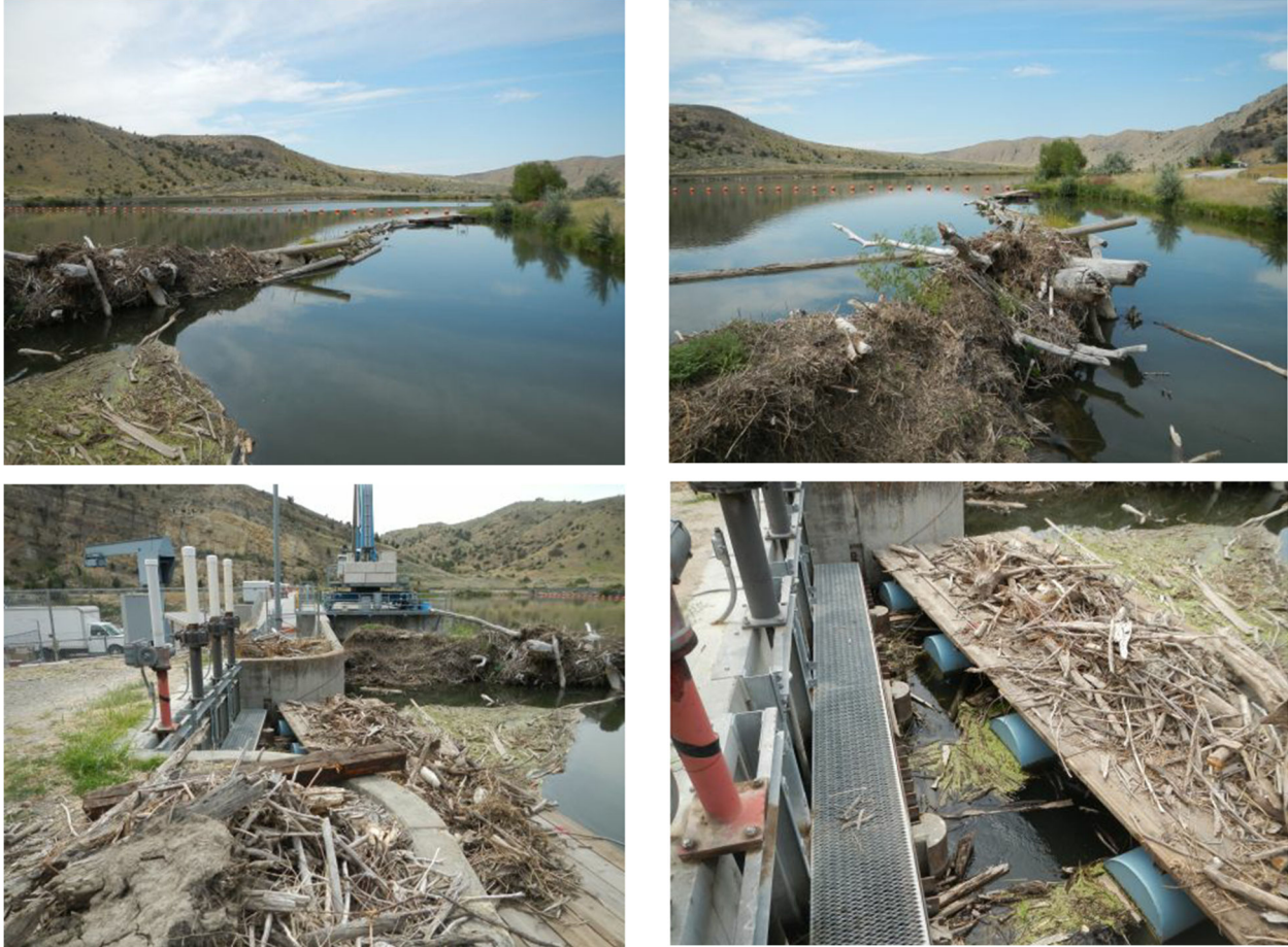
Figure 6: Representative Site Photos of the Existing Jetty and Irrigation Canal Headworks (photos taken July 2017)
