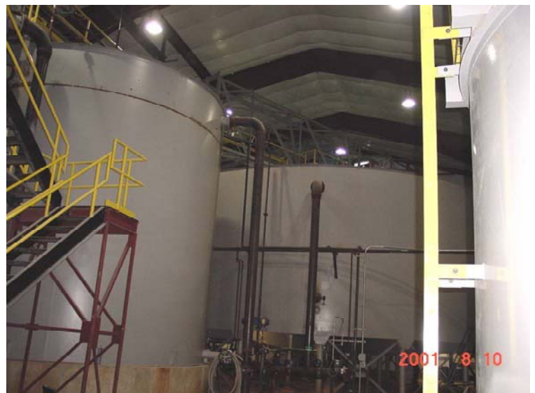
Inside the Landusky Mine Water Treatment Plant
