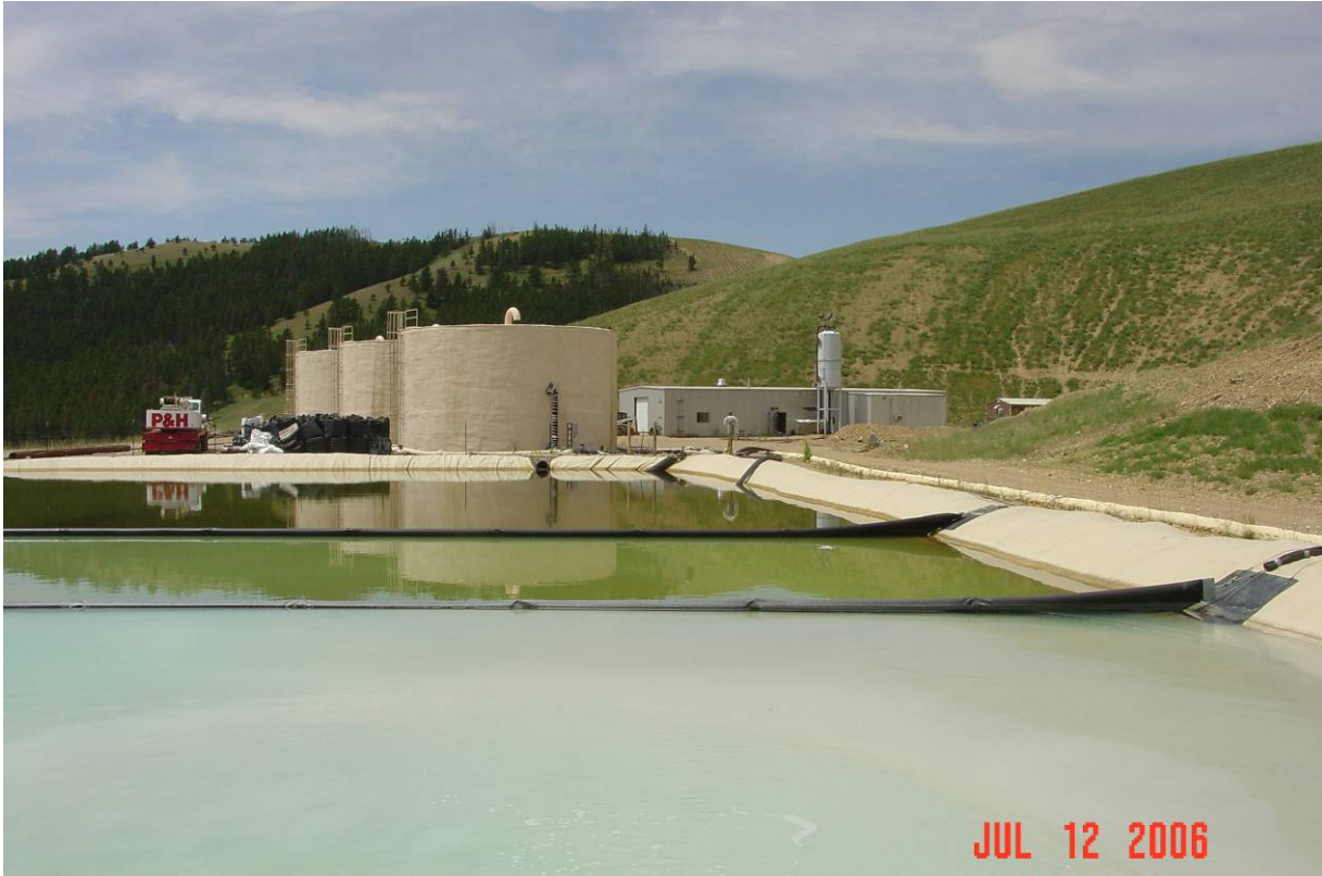
Bioreactor on the L87 Leach Pad Dike, pH pre-treatment pond in the foreground.
