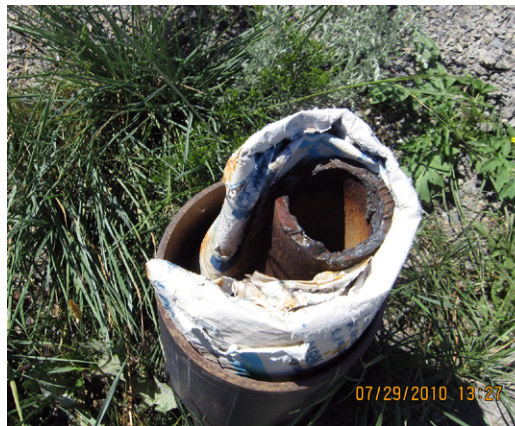
Improperly abandoned well
