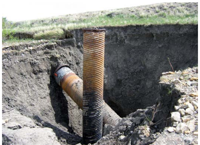
Recent failure of Petroleum County corrugated metal pipe
