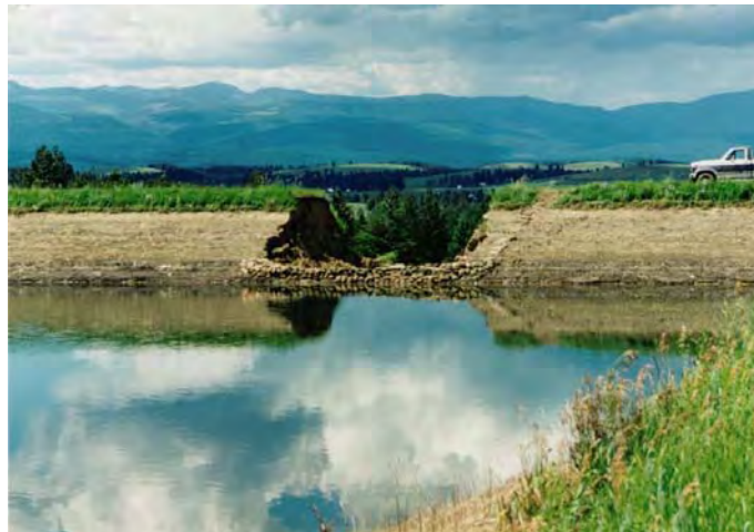
FIGURE 2. PHOTOGRAPH OF AN EARTHEN DAM BREACH IN MONTANA WITH VERTICAL BREACH SIDE SLOPES
