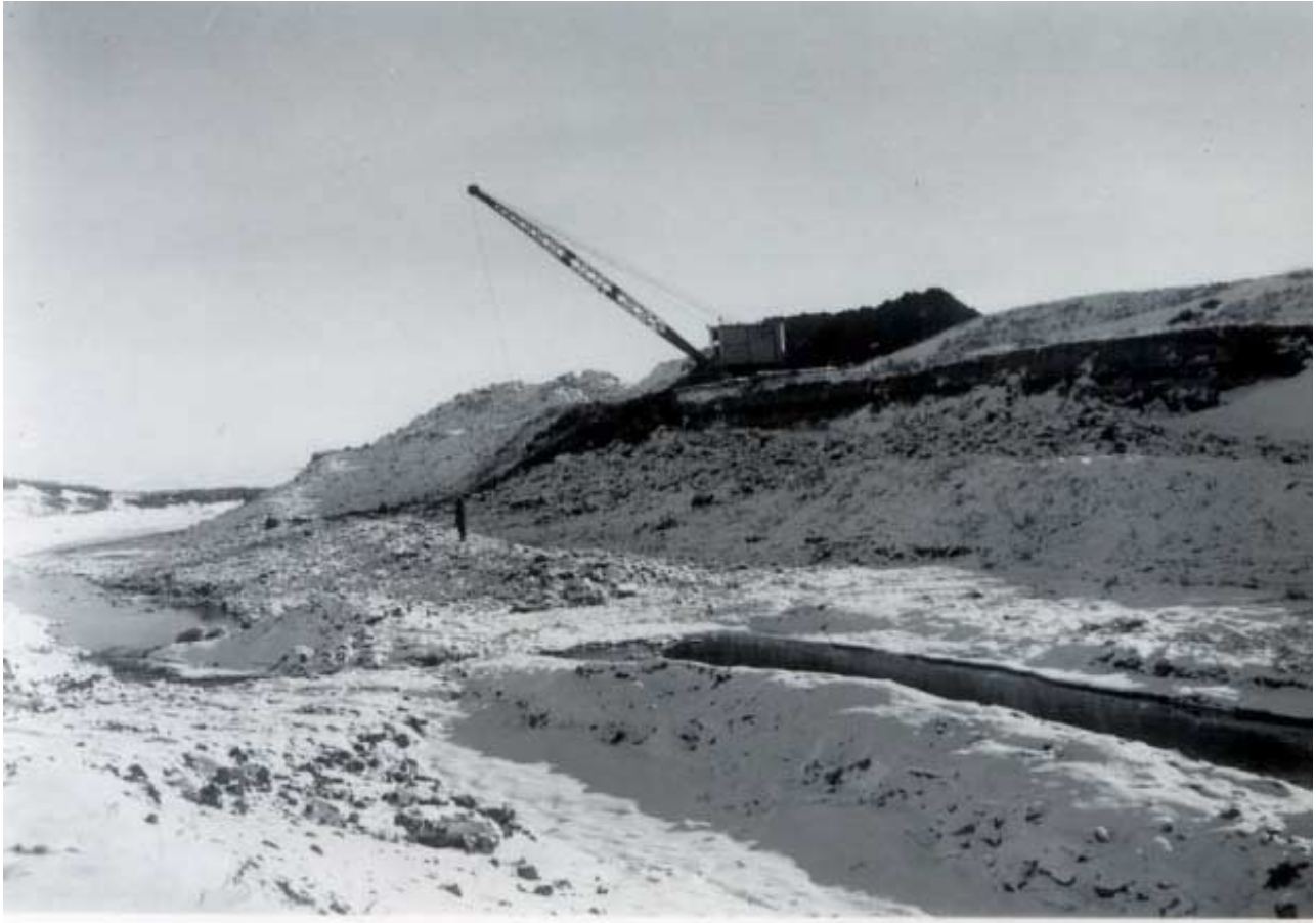
Dragline clearing slide material from St. Mary Canal. Circa 1952 - Courtesy of USBR
