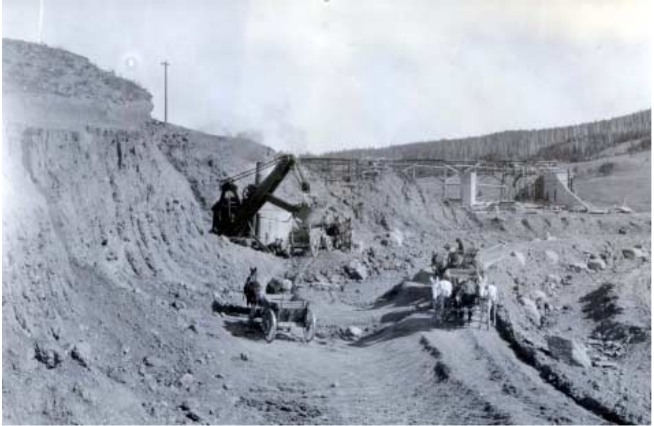
Steam Shovel and construction crews at work during construction of Sherburne Dam. Circa 1915 - Courtesy of USBR
