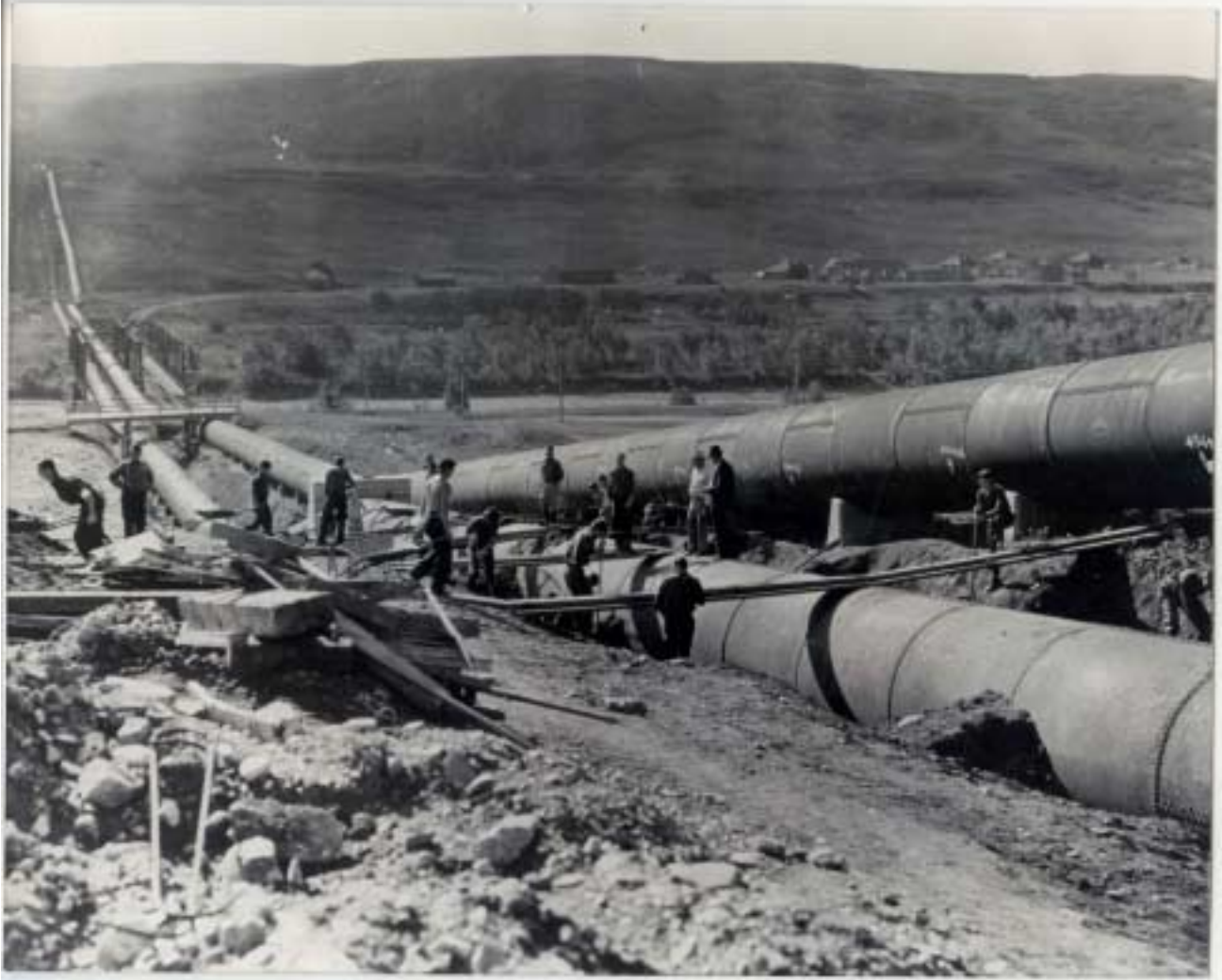
Repair work on left barrel of St. Mary River siphon. The Bureau of Reclamation's "Camp 9" in background. Circa 1930's - Courtesy of USBR
