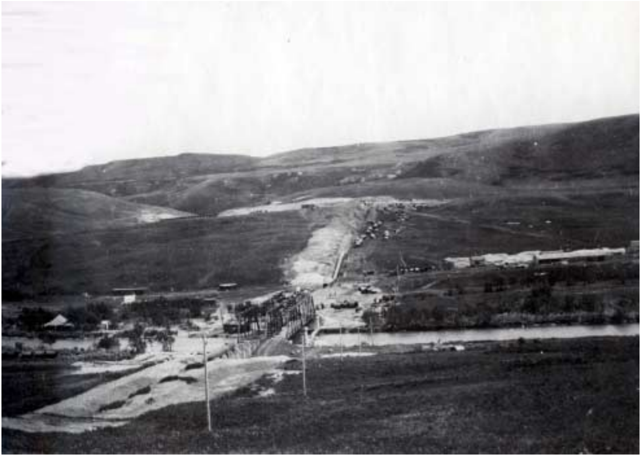
Construction of St. Mary River siphon; each siphon is 90 inches in diameter & approximately 3,200 feet long. Circa 1912-1915 - Courtesy of USBR
