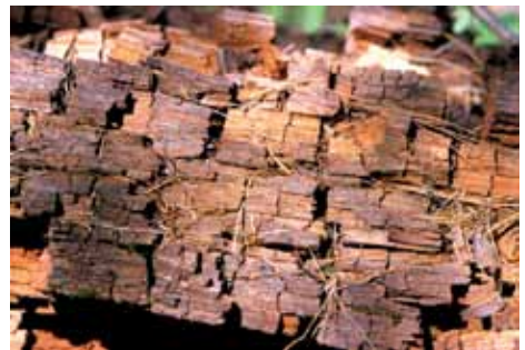
Figure 3. Advanced brown cubical decay caused by velvet-top fungus.
