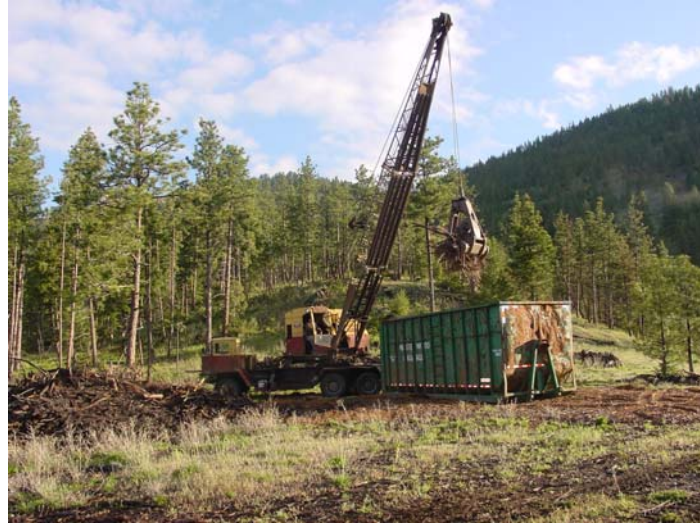
Figure 6. Crane loading a roll on/off container. The Bucyrus-Erie 22B Transit crane was equipped with a locally-manufactured cable grapple. The crane had a 40-ft boom which allowed it to reach down over steep road embankments.
