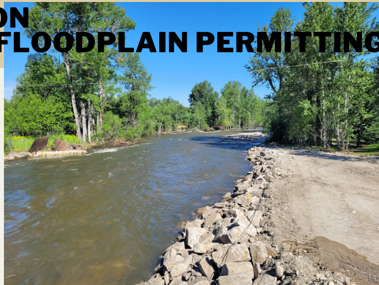
Riprap placed along the East Rosebud River bank after flooding and bridge repairs on Hwy 419 near Absarokee to restore access to Fishtail and Nye likely triggered emergency permitting. Photo by: S. Wingard (June 2022)
