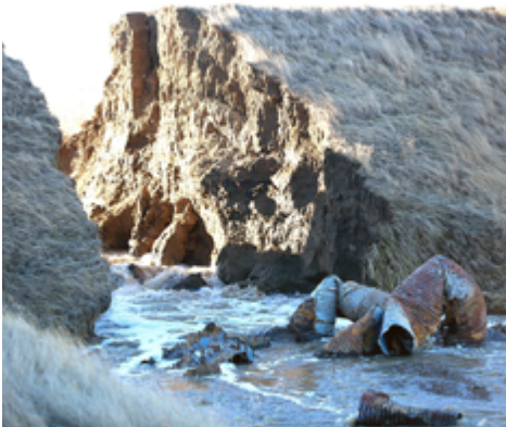
Chouteau County dam that failed in 2011
