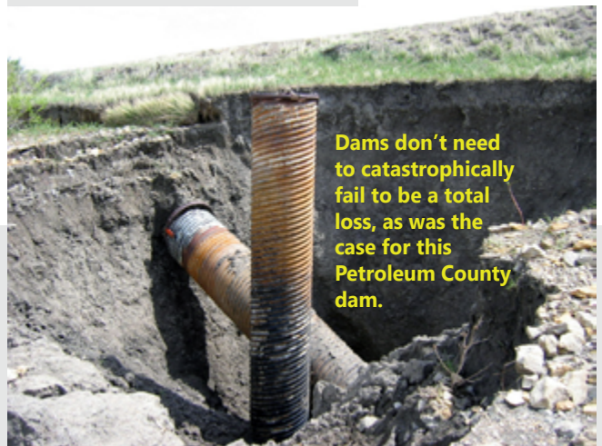
Petroleum County dam in distress
