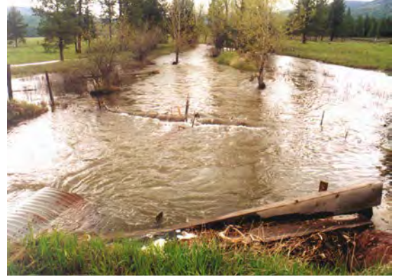
This undersized culvert caused large amounts of gravel to deposit in the channel upstream. Woody debris must be cleaned frequently from the inlet.
