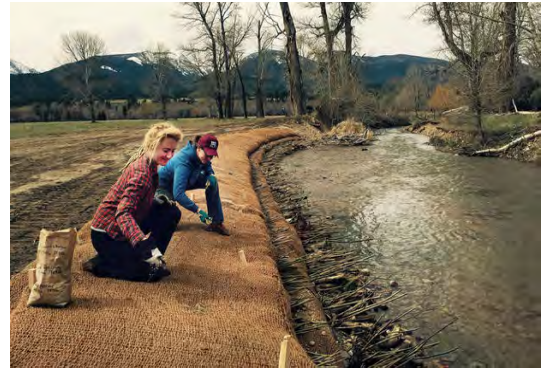
Soil lifts are commonly installed as a single or double layer ranging in thickness from 1 to 2 feet in depth.
