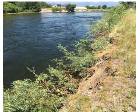
This bioengineered bank is deforming as the river undercuts the encapsulated soil lifts. Deformable banks are frequently incorporated into restoration strategies, but may be undesirable for structural protection.
