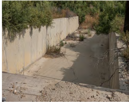
Dam spillway structures are commonly large rock or formed concrete and should be designed to withstand expected flood flows.
