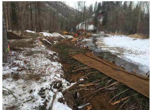
(Left) Aerial view and proposed treatment of avulsion (Above) Bank stabilization under construction
