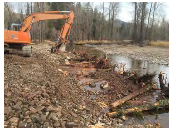
Large woody debris foundations are typically backfilled with some amount of large rock and native fill for ballast.
