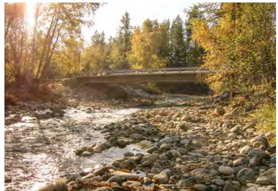
A well designed bridge spans the bankfull channel width (or more) and allows sufficient clearance for passage of flood, ice, and debris.
