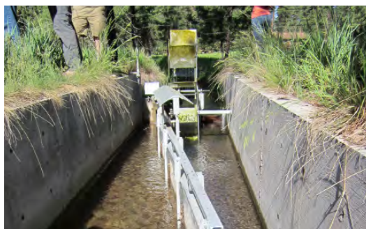
Fish screens are effective for preventing fish loss in irrigation ditches. A by-pass channel is normally needed to redirect fry to the main channel. A flat screen relies on brushes to clear debris.
