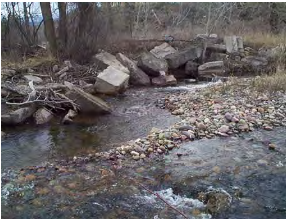
Concrete is generally not acceptable for large angular rock rip-rap. Contact Montana DEQ for guidance regarding use of concrete as rip-rap.
