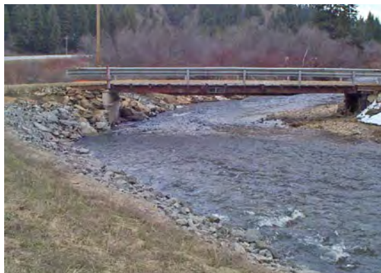
This bridge is set slightly above bankfull, but does not have wingwalls. Location on a meander is not ideal, although upstream rip-rap limits lateral movement. Note, point bar is still growing under bridge.
