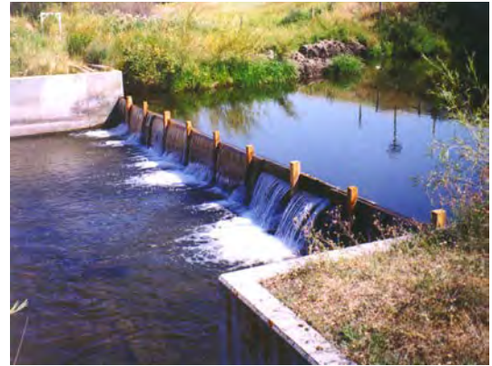
Concrete may be preferred to wood for longevity. This structure is not fish friendly because of the height of the drop and the flat slab downstream.
