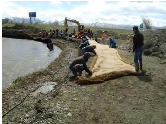
Bioengineering treatments can be labor intensive, especially for installation of fabric. Bioengineering is preferred where vegetation treatments can be successfully established.
