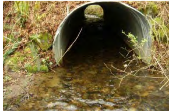
Pipes must be designed to retain bed material. This generally requires sizing the pipe not just for hydraulic capacity but to accommodate flood events and retain bed material in the pipe.
