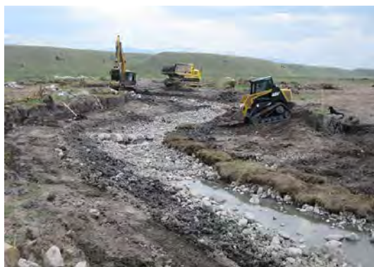
Ideally, in stream work can be completed “in the dry” by diverting or pumping water around the site.
