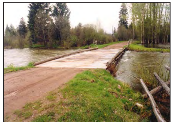
This bridge stringer is also a good indicator of bankfull. Projects should avoid this situation, which traps debris.
