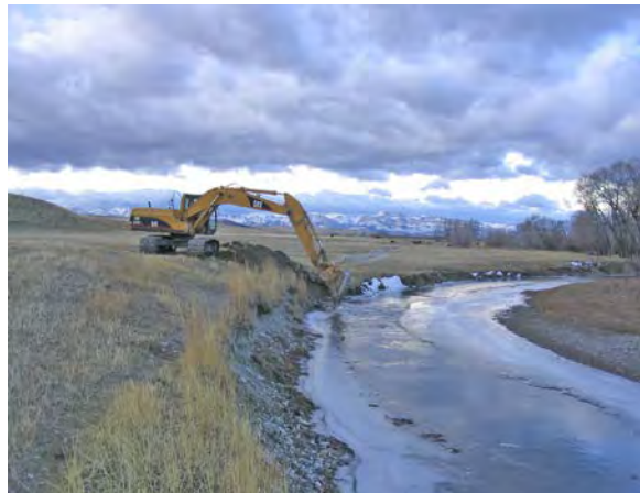
Construction activities on the bed and banks of perennial streams generally require both state and federal permits. No floodplain permit was required for this project.
