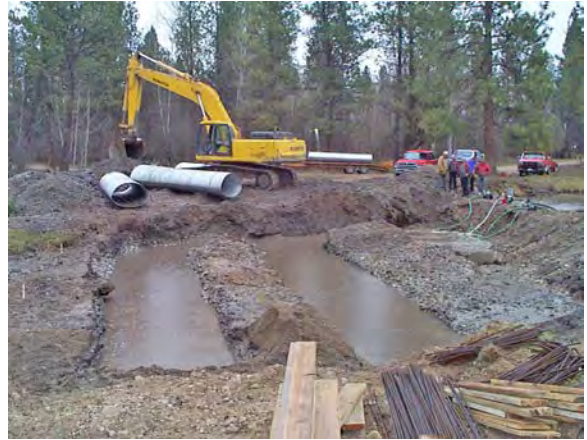
Dewatering construction areas with pumps requires a MPDES permit when discharging to State waters.
