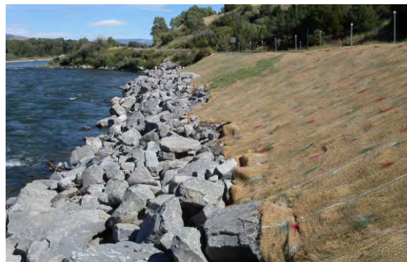
An engineered rip-rap bank provides a high degree of protection, but diminishes natural river and aesthetic values. These can be enhanced by incorporating vegetation above high water mark.
