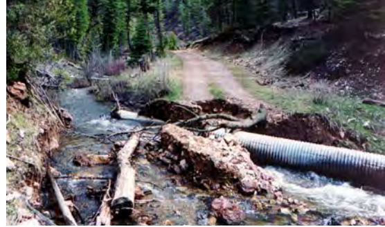
Undersizing pipes to save money is a poor strategy.
