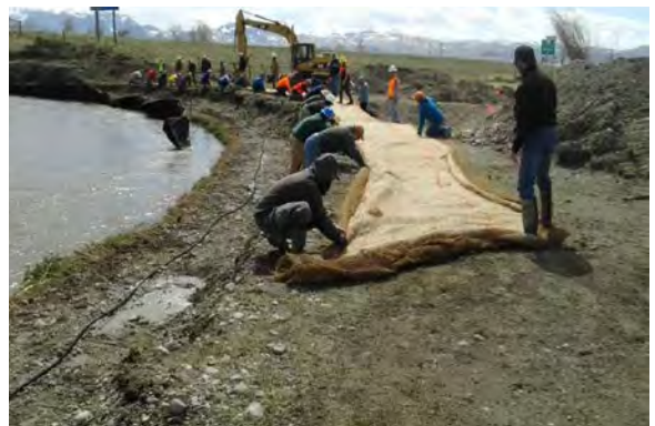
Geotextile bank treatments can be labor-intensive. Backfilled brush layer in place, ready for first soil lift.
