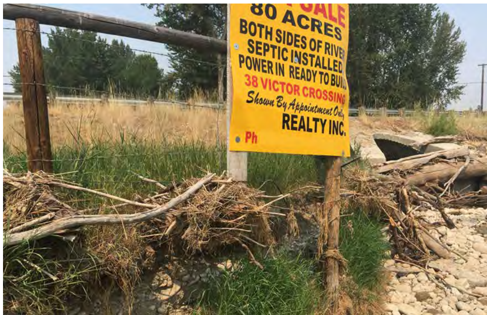
Although floodplain permitting can be time consuming and costly, the process helps ensure that existing and future development minimizes risk of flooding problems. Note the high water mark/debris at the base of the sign.
