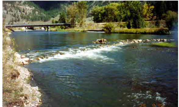
One of the structures at left, prior to failure. The warning signs were apparent, notably the elevation of apex above the bed, and 2-ft + high drop over the flat sill.
