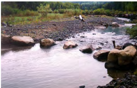
True "V" weirs generally have a row of cap rocks with spaces, rather than a flat sill. This promotes bedload passage (to some extent), but does not always work well for irrigation diversion needs.
