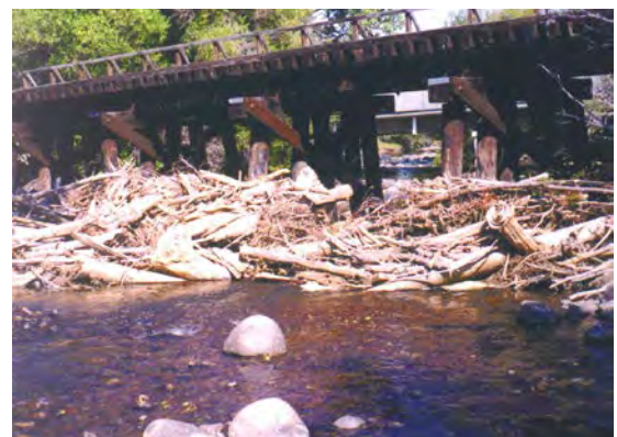
Debris jams are often associated with center piers on bridge crossings. A clear span is preferable to piers.
