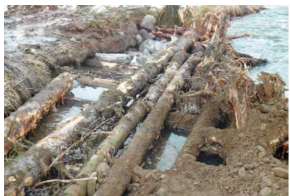
A robust toe protection technique relies on large woody debris to provide a high degree of scour protection.
