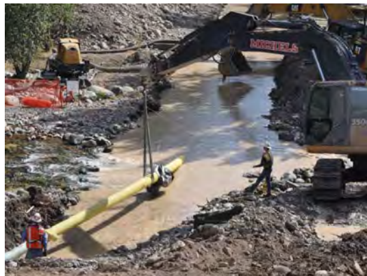
Flowing water through a construction site can result in severe water quality impacts. Potential sediment release must be addressed during the permitting process.
