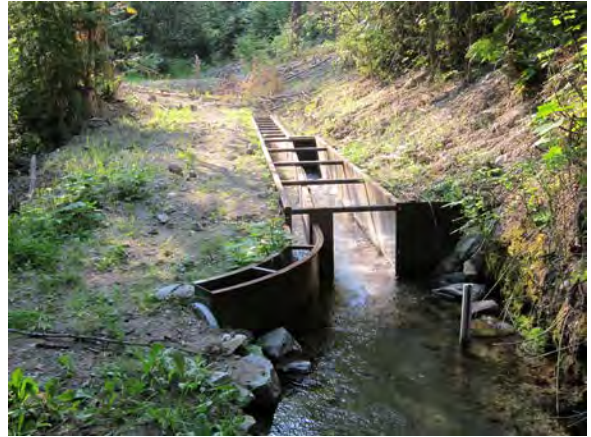
The screen entrance is in the background; foreground shows screened water on the right and bypass channel (fish return) on the left.
