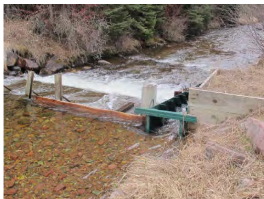
Original stopboard structure and Denil ladder did not provide adequate fish passage.
