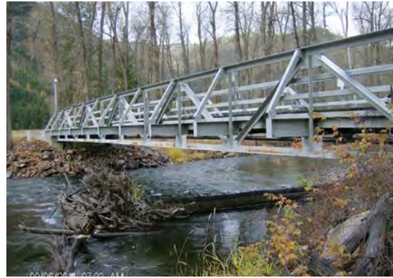
This well-designed bridge has adequate clearance for ice, debris, and peak flows. Note, however, that the abutments do encroach on the channel somewhat.
