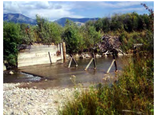
Wooden diversion structures have a limited life but are easily constructed. These type of diversions often form fish barriers because of the stopboards and flat floor.
