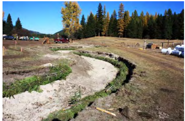
In moderate scour or erosion applications, toe protection can include brush layers, fascines, and small woody debris.
