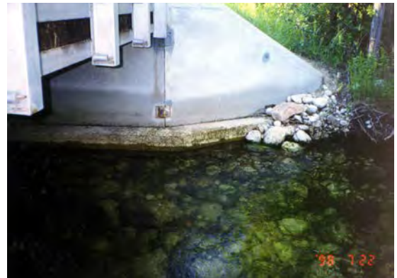
Concrete can make good abutments, provided the footing is placed below scour depth. This footing should be 2 feet lower.
