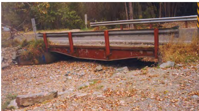
A low stringer in an aggrading channel does not leave much room for water. Note that the beam hangs low in the center and restricts peak flow capacity and debris passage.
