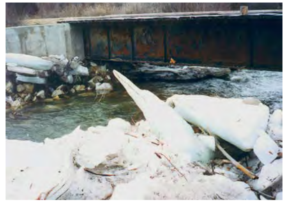
This bridge stringer was set below bankfull, and had problems with ice jams and flow capacity.
