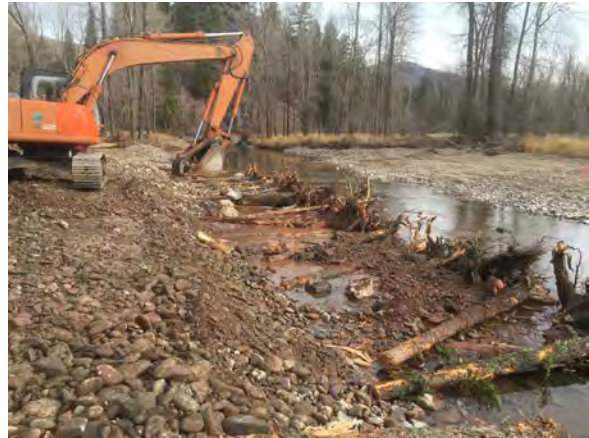
Root wads and woody debris can provide substantial bank protection while enhancing fish habitat. Large wood can serve as robust toe protection or incorporated into the entire bank.
