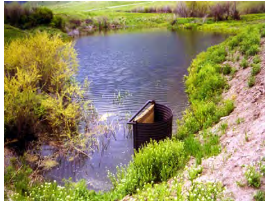
Canal checks are commonly used on small ponds to control water elevations. Canal checks and standpipe structures do not substitute for emergency spillways.
