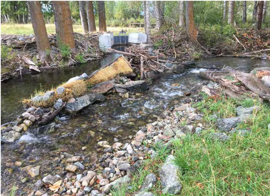
Older diversions that require maintenance or reconstruction offer opportunities for improvement in terms of functionality, fish passage, and stream function.
