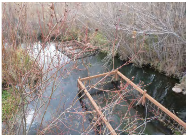
Beaver deceiver™ installed at upstream end of culvert to prevent beaver from damming.
