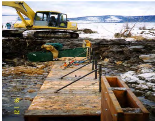
The flat floor and high drop of a pin and plank structure limits fish passage.
