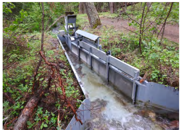
Fish screens on diversion structures prevent the loss of fish in irrigation ditches (entrainment)
