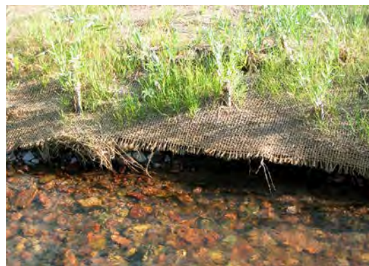
Biodegradable geotextiles can last 2 to 4 years while vegetation becomes established. Note, however, that the fabric in this photo has been abraded in the first year. Ultimately, all biodegradable fabric treatments rely on vegetation for long-term stability.
