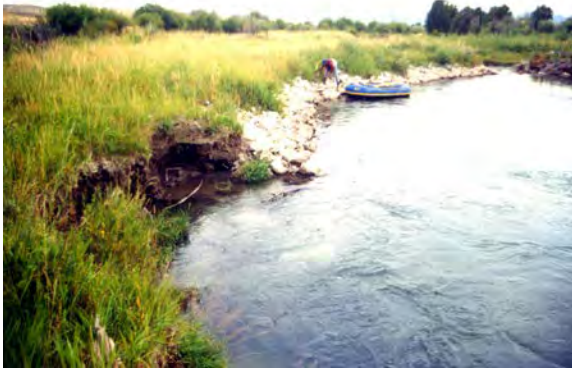
Receding bank upstream of a rip-rap job will eventually lead to failure.
