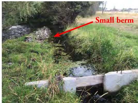
Small temporary berms may be appropriate in some locations as a low-impact alternative to permanent structures.
