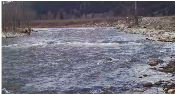
Large weirs must frequently be built in series to avoid large drops exceeding structural stability. Construction of weirs in high bedload transport streams always carries some risk of failure.
