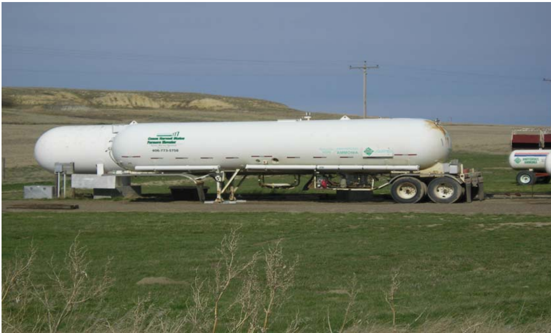
Unsecured Anhydrous Ammonia Tanks in Richey
