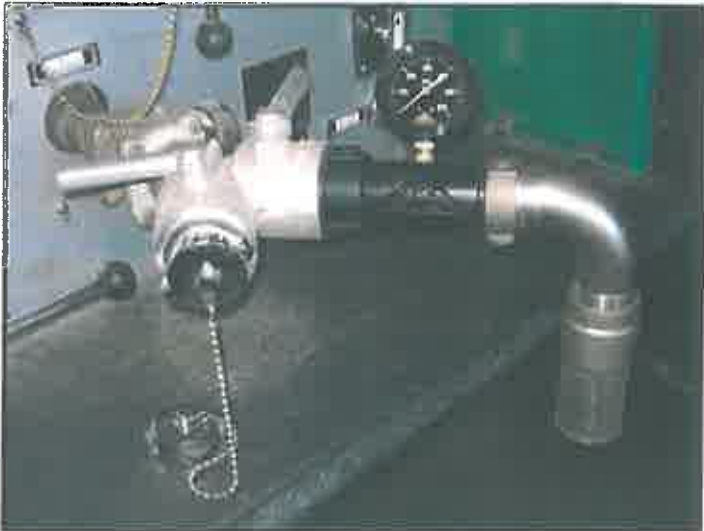
Figure 3. Pressure valve attached to the footvalve.
